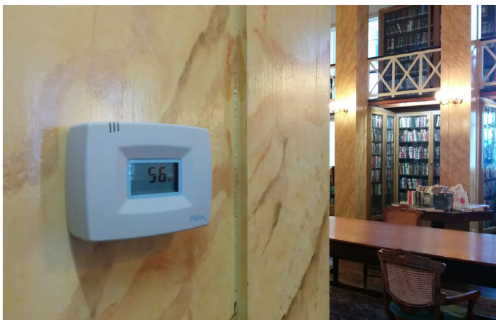
Preservation Environment Monitor (PEM) data logger in the Members' Reading Room.
